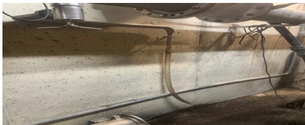
Photo of wastewater before treatment area
