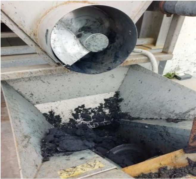
Sludge Sampling Point
