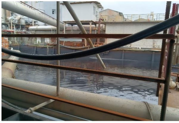
Photo of wastewater before treatment area
