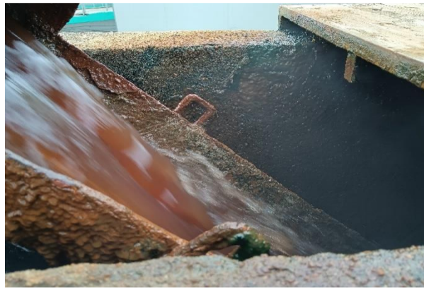
Photo of wastewater sampling point (after treatment)
