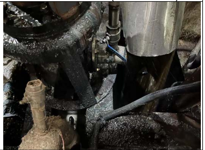
Untreated wastewater 2 (high concentration)
