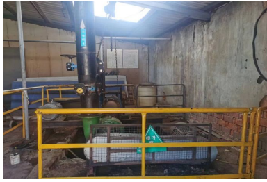
Photo of wastewater before treatment area
