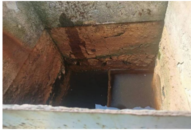
Photo of wastewater sampling point (after treatment)
