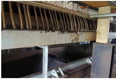
Photo of Sludge Area
