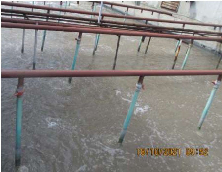
Foam in Aeration Tank
