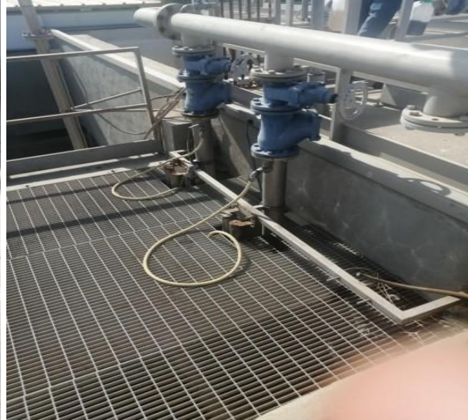
Raw Waste Water Sampling Point
