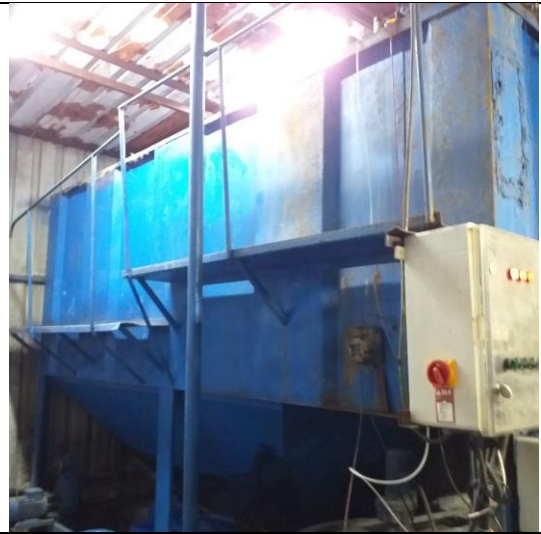
Panoramic view of treatment plant
