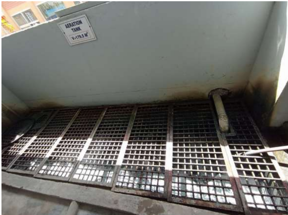
Pic- Foam in Aeration Tank
