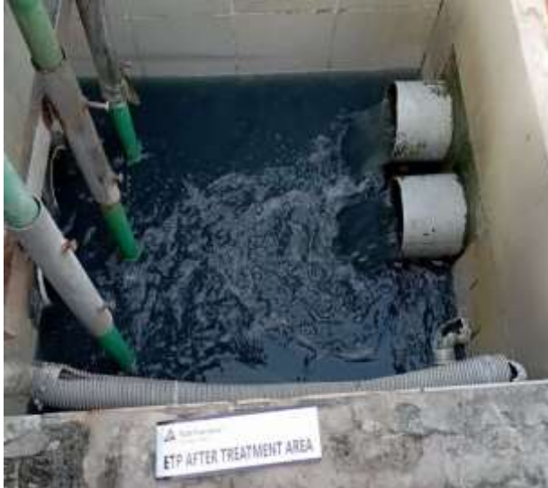
Photo of the Sample/Sampling Location M001- ETP outlet water (After Treatment)
