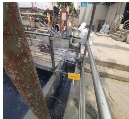
Sampling point - Raw Wastewater
