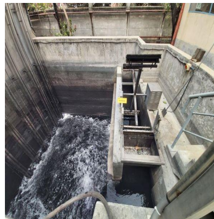
Sampling point - Raw Wastewater
