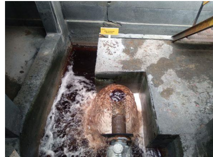
Photo of after treatment area
