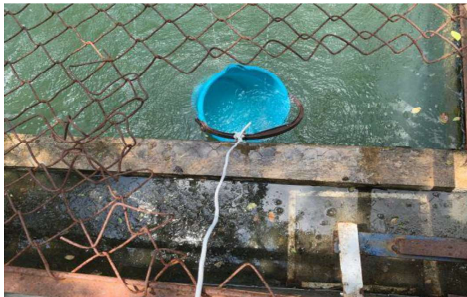
Treated Wastewater Collection Point
