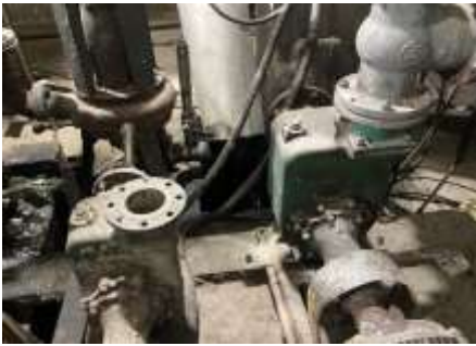
Photo of before treatment area (High concentration)
