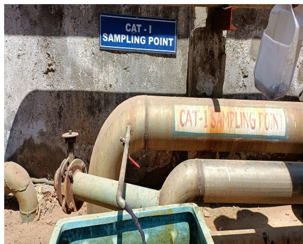
Photo of sampling point Sample -3 (Raw Wastewater-Low TDS (Unit- 3))
