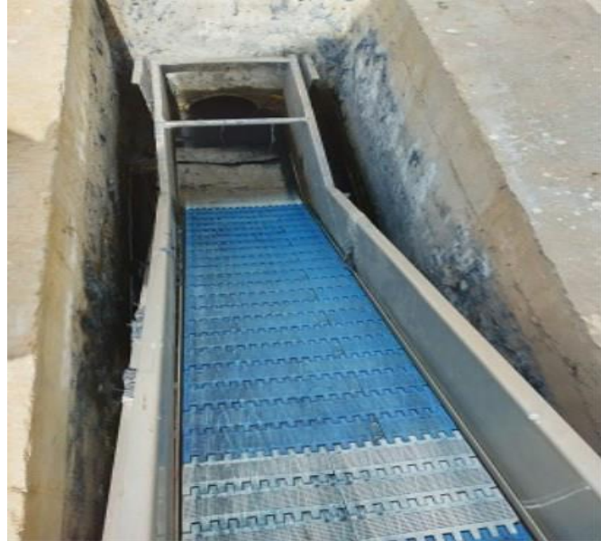
Raw waste water sampling point
