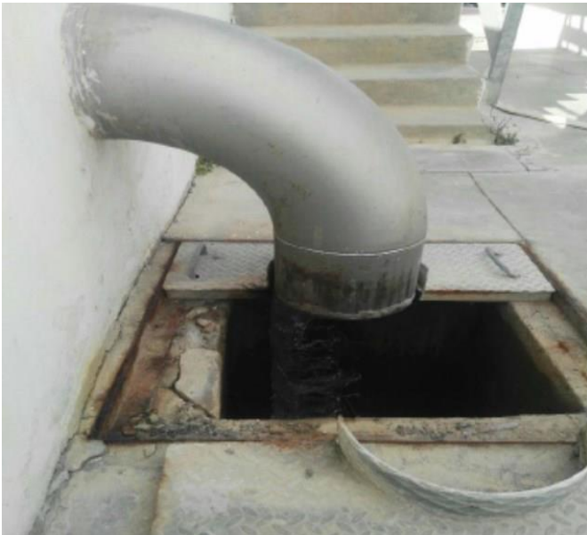
Discharged Wastewater Sampling Point
