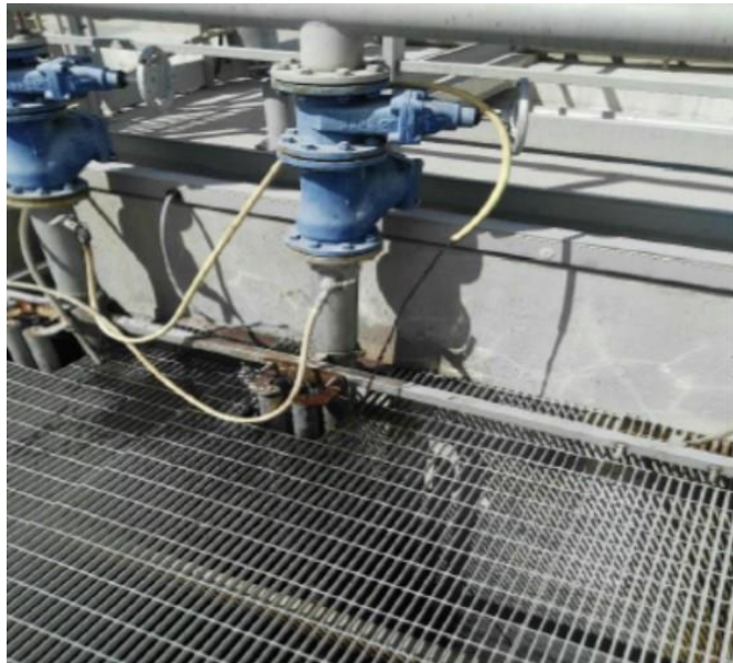
Raw Wastewater Sampling Point
