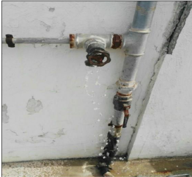
Incoming Water Sampling Point
